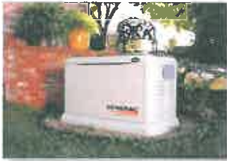
Automatic standby generator
